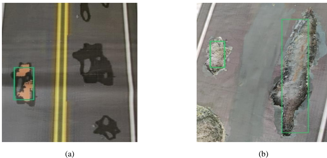
Fig. 6 Detected Figure (a) Top View potholes detection (b) Area mapping potholes
