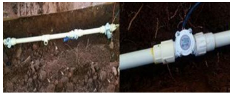
Figure 2: Real-time Water flow sensor placement
